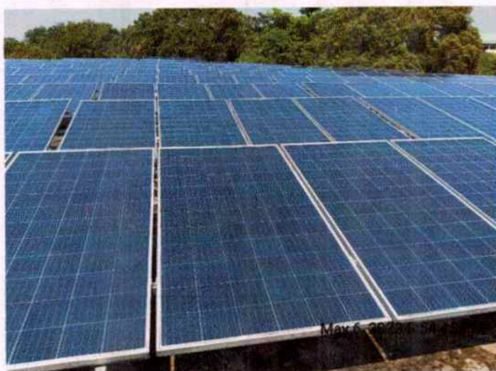
View of Installed Rooftop Solar Panels
