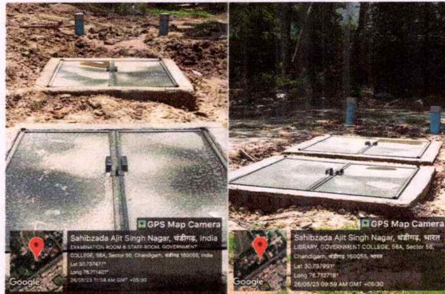
Photo 59: College's Rainwater Harvesting System
