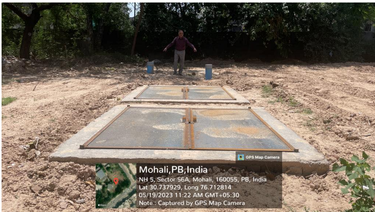
(Fully Functional Rainwater Harvesting System)
